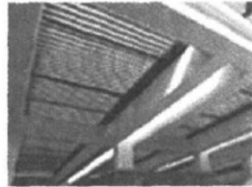
Solar heat collecting pipe installed on the roof.
